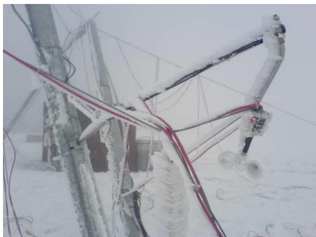
Figure 4-1: A collapsed meteorological tower, likely due to heavy icing.
