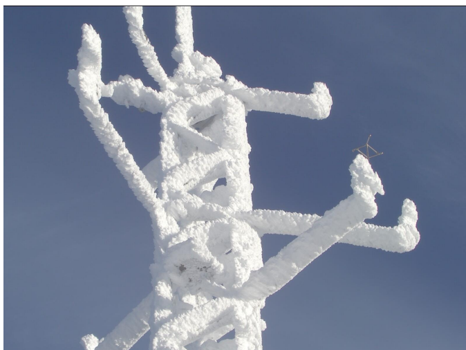
Figure 4-2: The impact of ice build-up on mounting hardware and sensors must be considered to ensure the accuracy of wind speed and direction measurements. Photo credit: TMV2 Murdochville, TechnoCentre éolien.
