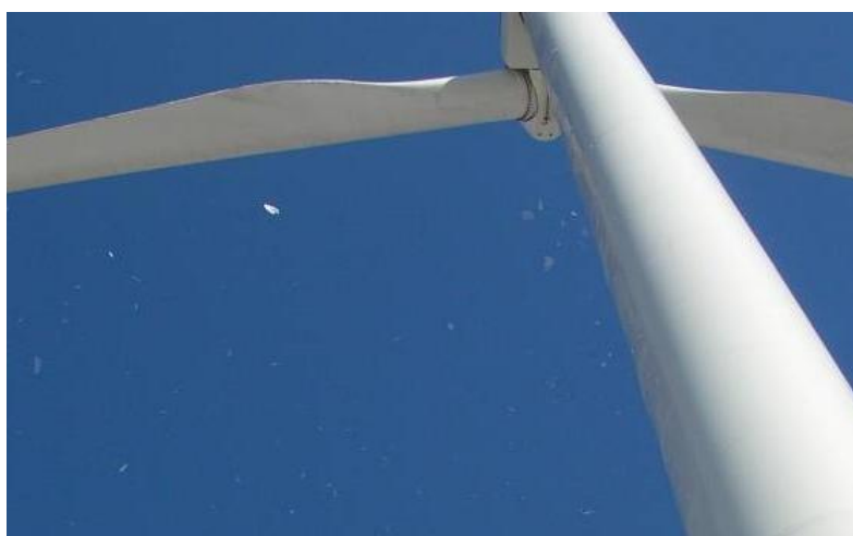
Figure 8-2-1: Ice falling or being thrown off a wind turbine poses a safety threat to turbine maintenance staff and, depending on turbine siting, the general public. Photo credit: Jeroen Van Dam, USA
